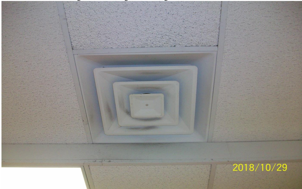
#2 – Room 135 – Ceiling ventilation register with light dust.
