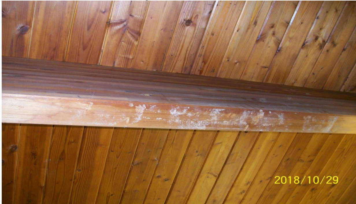
#1 –Room 132 – Wood Paneled Ceiling Joist with dust.
